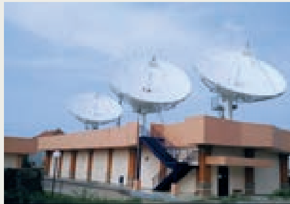
Backup Satellite Control Facility (BSCF), Bali
